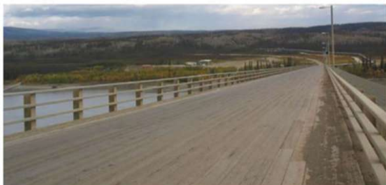
▲ This photo shows both the Yukon River bridge's wooden deck, and the grille along the right side covering the pipeline. (August 2004, courtesy of Walter Haight)
